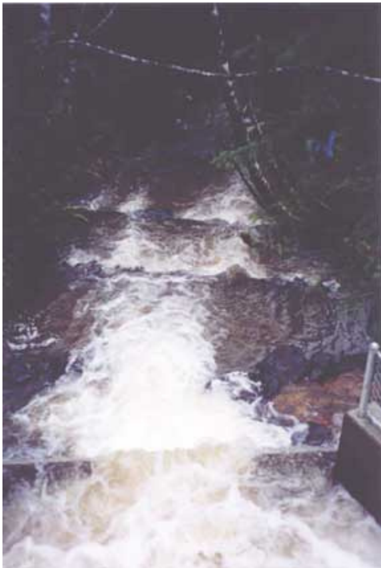
Looking downstream at jump pool weirs. Top weir not intact. 02/02/99
