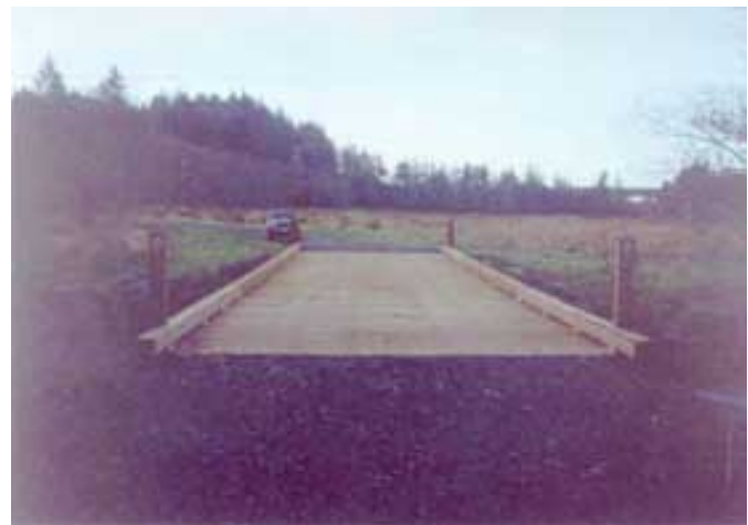
Looking at the bridge decking (notice no running boards)
