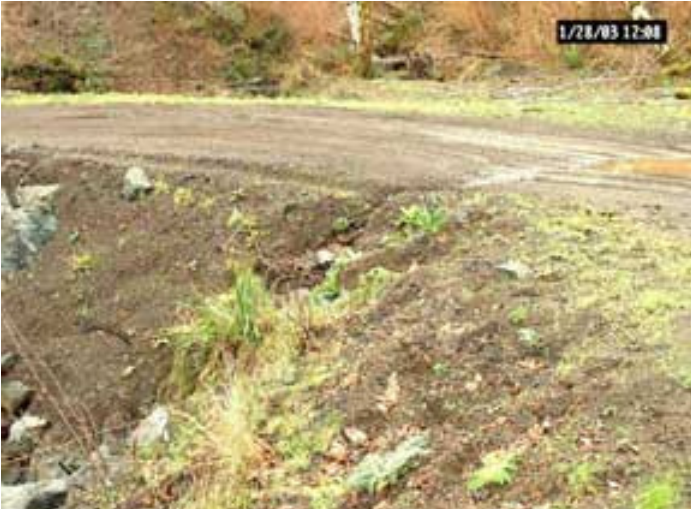
knox 1 mp 1.130 Runoff mining road fill
