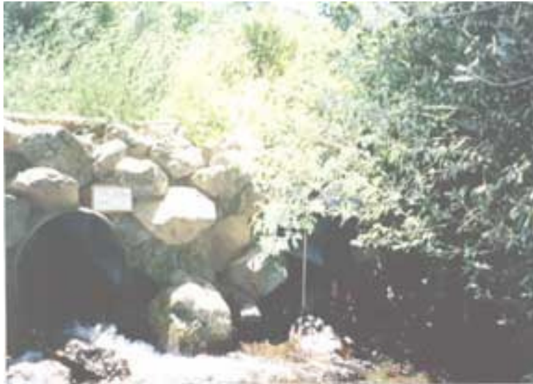
Outlet of former crossing – acting as a complete blockage during summer flows
