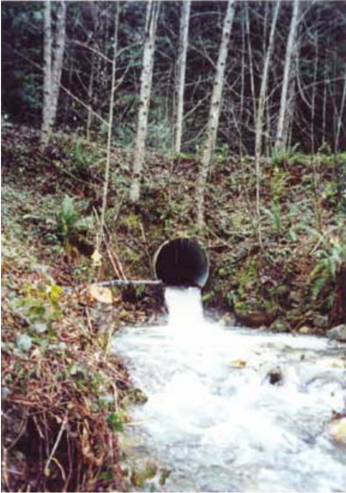
Another barrier with 3-4' drop, upstream on a private road
