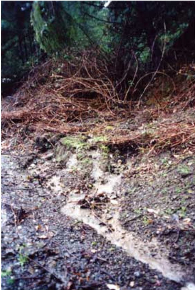
Exposed fill adjacent to inlet eroding during rainstorm
